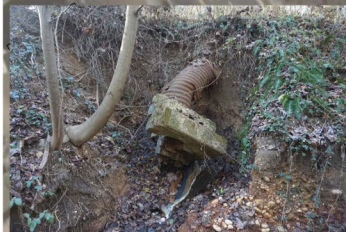
Existing Failed Pipe (Photo: Straughan Environmental, Inc.)
