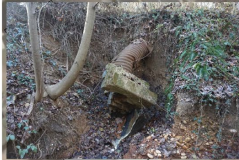
Existing Failed Pipe (Photo: Straughan Environmental, Inc.)
